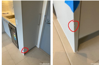
#596 | Level 03 > 49 > Entry | Cabinet Maker Edge strip is damaged at base of electrical cabinet
