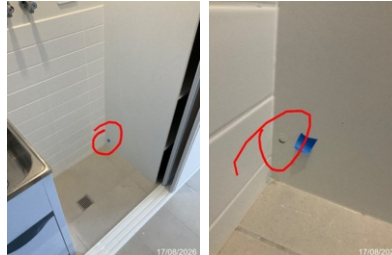
#595 | Level 03 > 49 > Laundry | Cabinet Maker Screw cover at base of shelving gable does not cover screw
