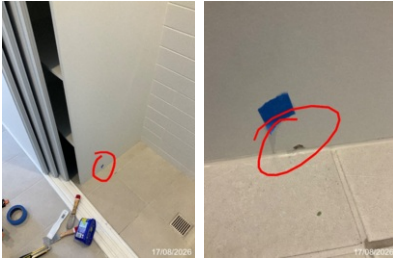
#628 | Level 03 > 48 > Laundry | Cabinet Maker Touch up chip at base of shelving gable
