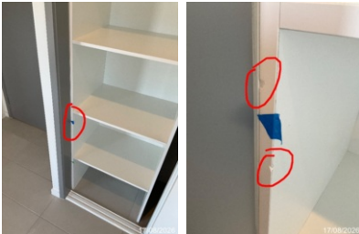
#610 | Level 03 > 49 > Bed 1 | Cabinet Maker Shelving left edge strip is damaged in 2 locations
